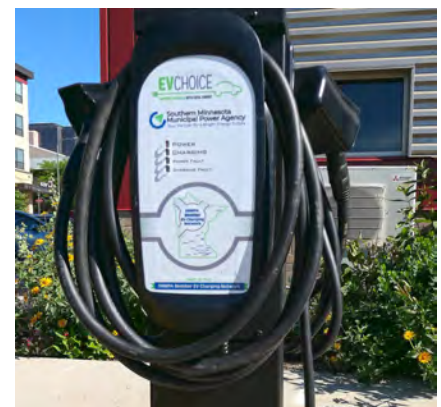
SMMPA's Level 2 Charging Station
