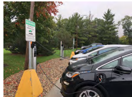
MNSU's Charging Infrastructure
