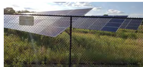
Connexus Energy Solar Garden
