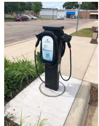
Available Level 2 Charging
